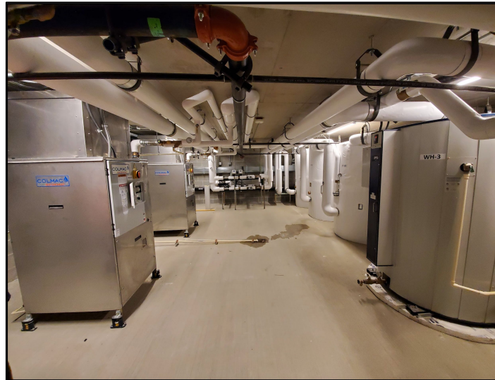
Large Commercial System
