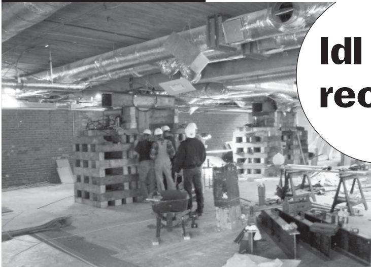
Above: view of structural repair work at the Lighting Design Lab. Problems with the building's foundation were uncovered during remodeling and had to be corrected immediately.
